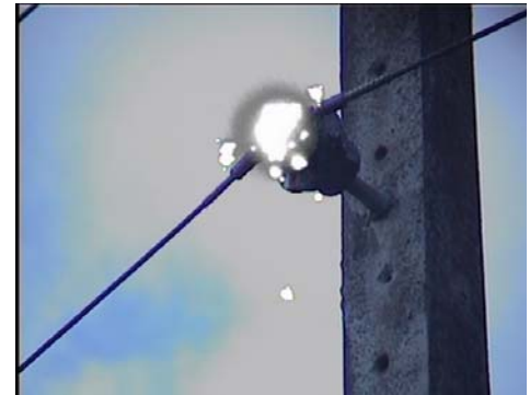
Figure 1: Insulator on 11 kV line with excessive corona
