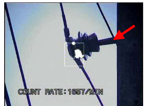
Figure 2: Insulator on 11 kV line with excessive corona
