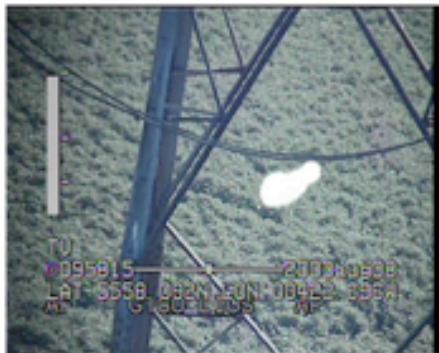
Corona discharge visible from broken conductor strand
