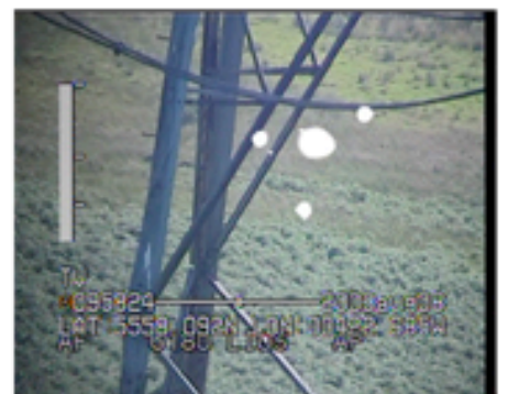
Broken conductor strand on 275kv dropper
