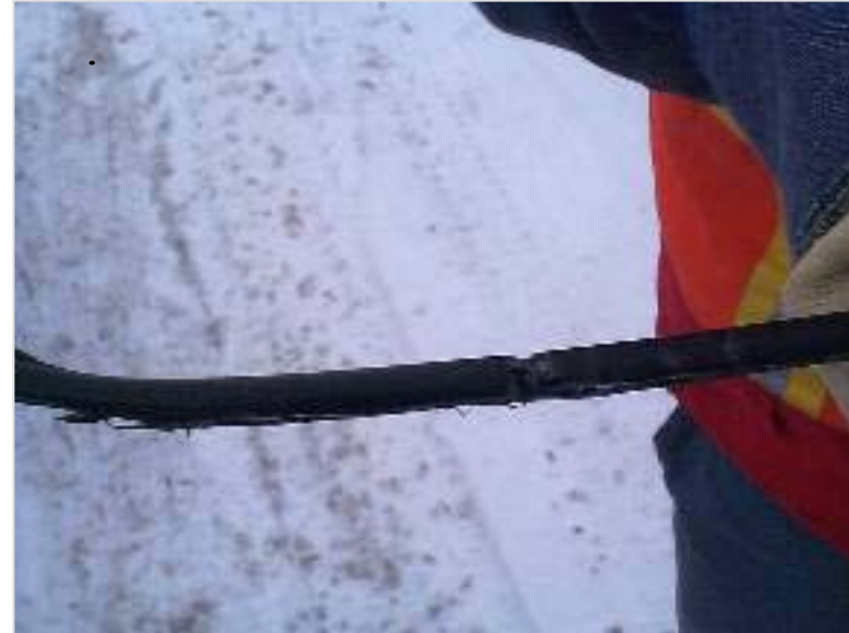
The rubber-covering on the 12.47kV wire: erosion of the rubber was caused by arcing on the 12.47kV wire that was attached to the pin insulator.
