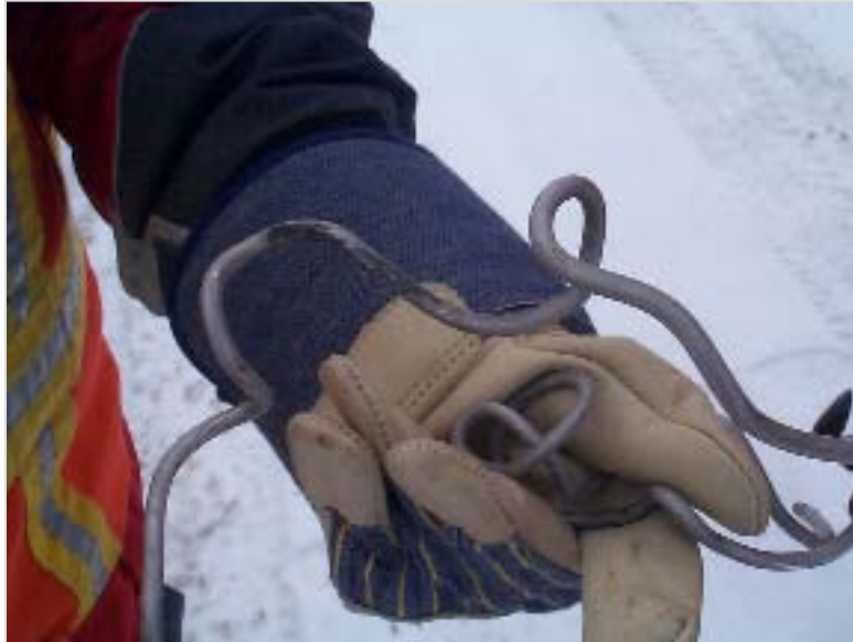
Flat spots on the aluminum tie wrap were found on on the 12.47 kV pin insulator .
