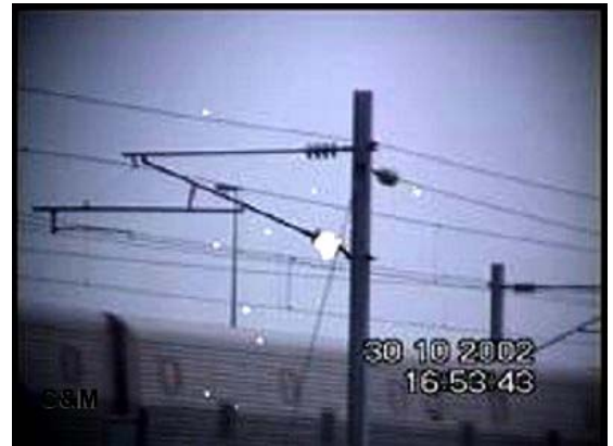
Figure 1: Note the strong discharge on the lower insulator of the pylon on the right side of the railway
