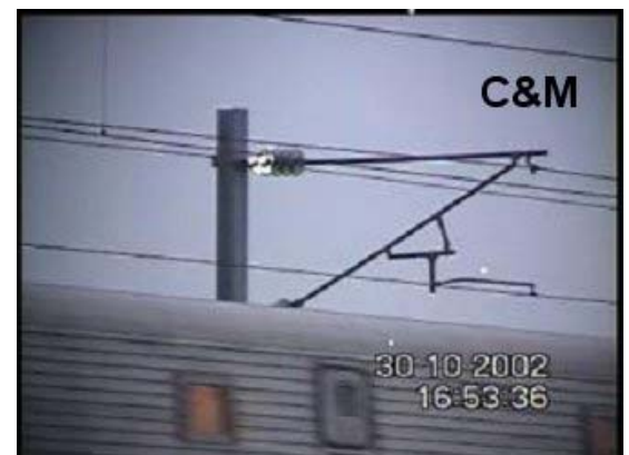
Figure 3: Corona on one of the insulators on the left side of the railway. This side was washed, the discharge on this insulator is due to either insufficient washing or the team skipped this insulator for unknown reason
