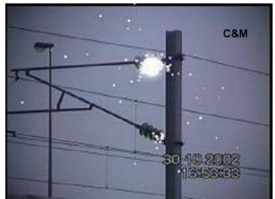
Figure 2: Pylon on the right side of railway. There is Corona on the lower insulator and arcing on the upper insulator. This side was not washed
