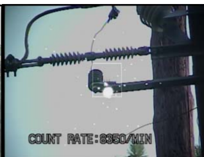
The exact corona arcing location
