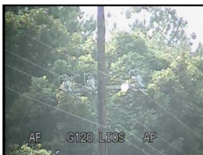
Arcing corona seen hundreds of feet away on hazy day.
